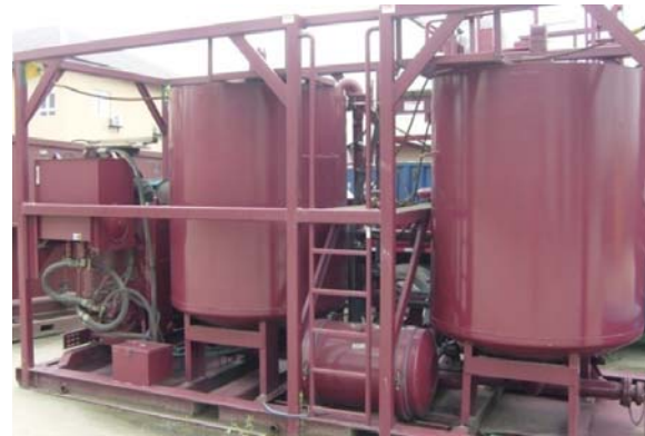
BATCH MIX UNIT
